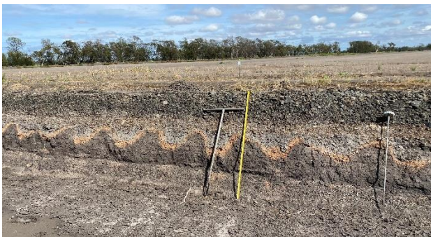
Figure 3. Photo showing typical plastic deformation of rail formation behavior during N2NS earthworks trial.
