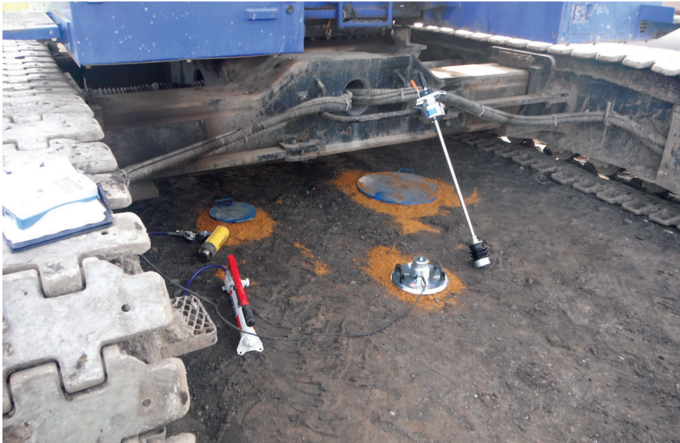
Figure 1: Attempts were made to find and map reinstated trial pits located within a piling rig plant yard
