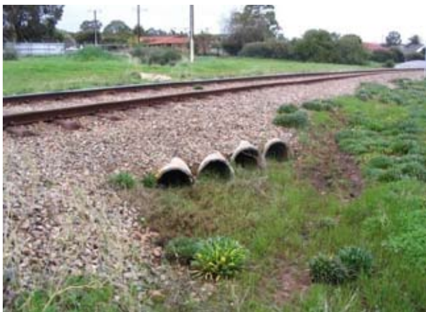
Figure 7: Poor drainage and blocked culvert
