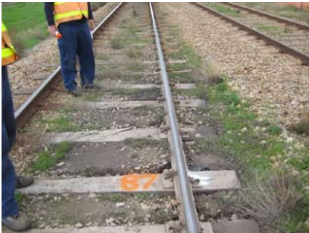
Figure 1: Walkover inspection with track pumping
