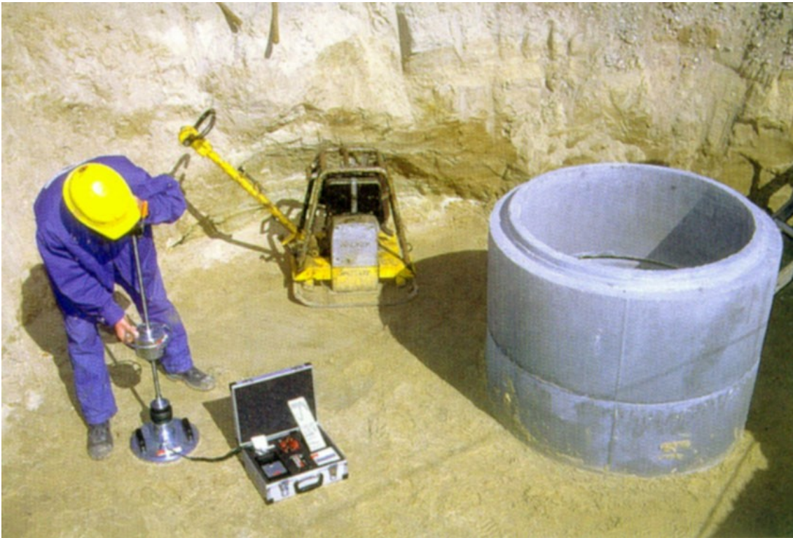
Figure 2: Dynamic plate load test using the Light-Weight Deflectometer according to TP BF-StB, Part B 8.3 in narrow conditions
