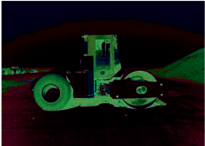
Ammann vibratory smooth drum roller with ACE system to output kB stiffness values: Field Study 2
