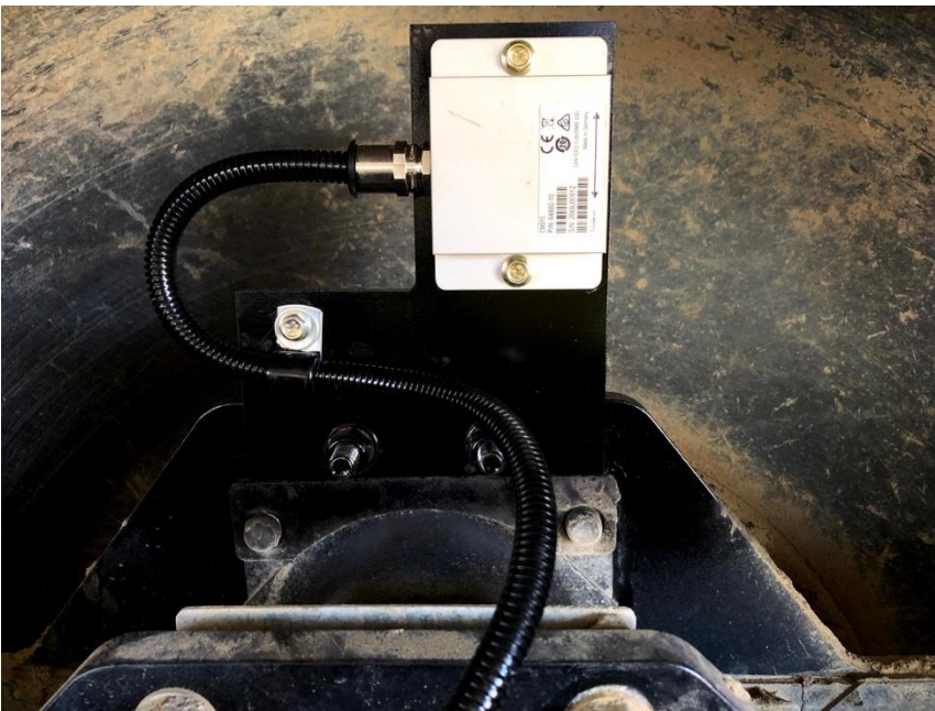
Figure 3.2 An accelerometer installation on the IC roller used in the compaction auditing trial
